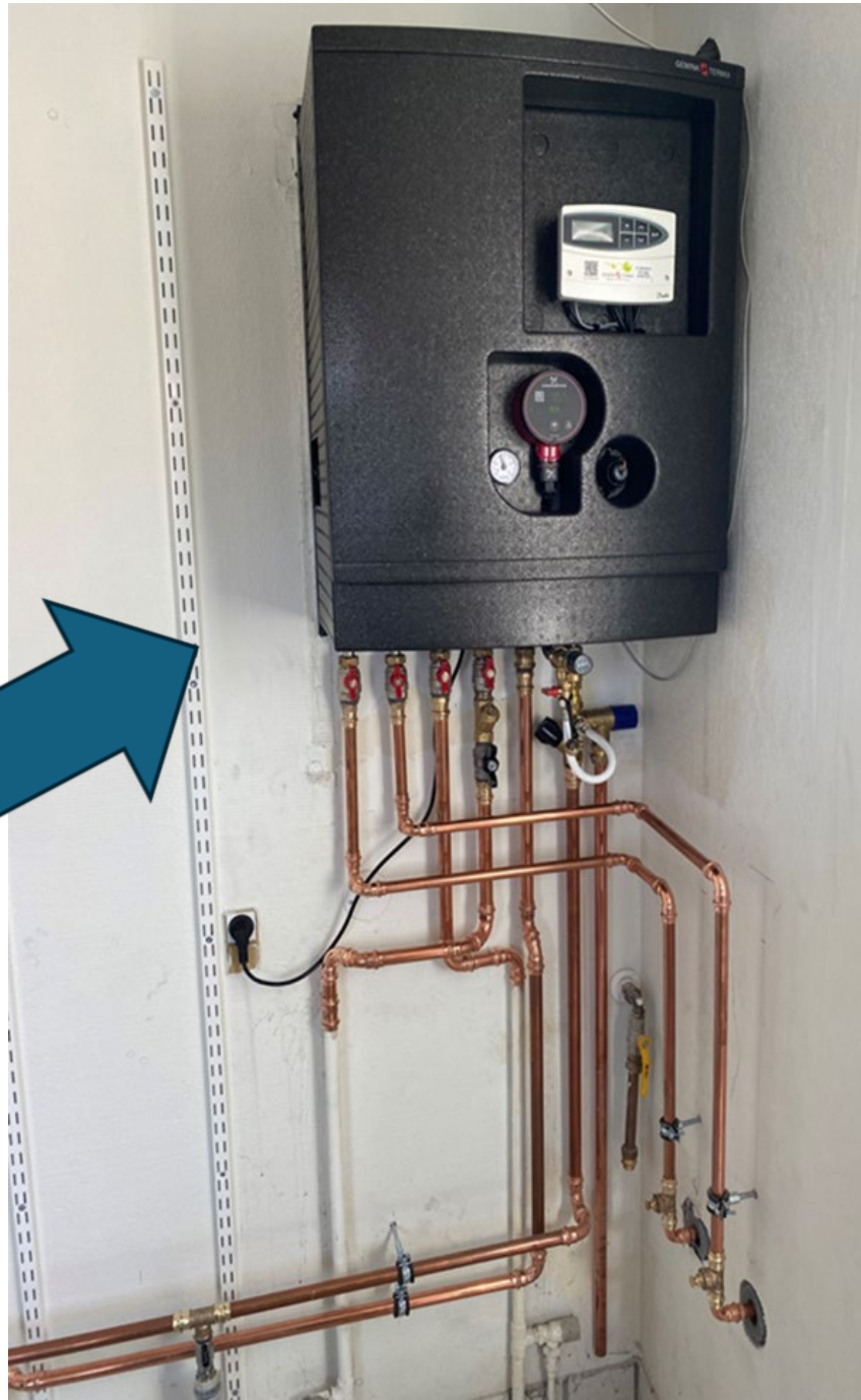
New compact Heat Interface Unit (HIU) NB. with bare pipework before it was insulated!
