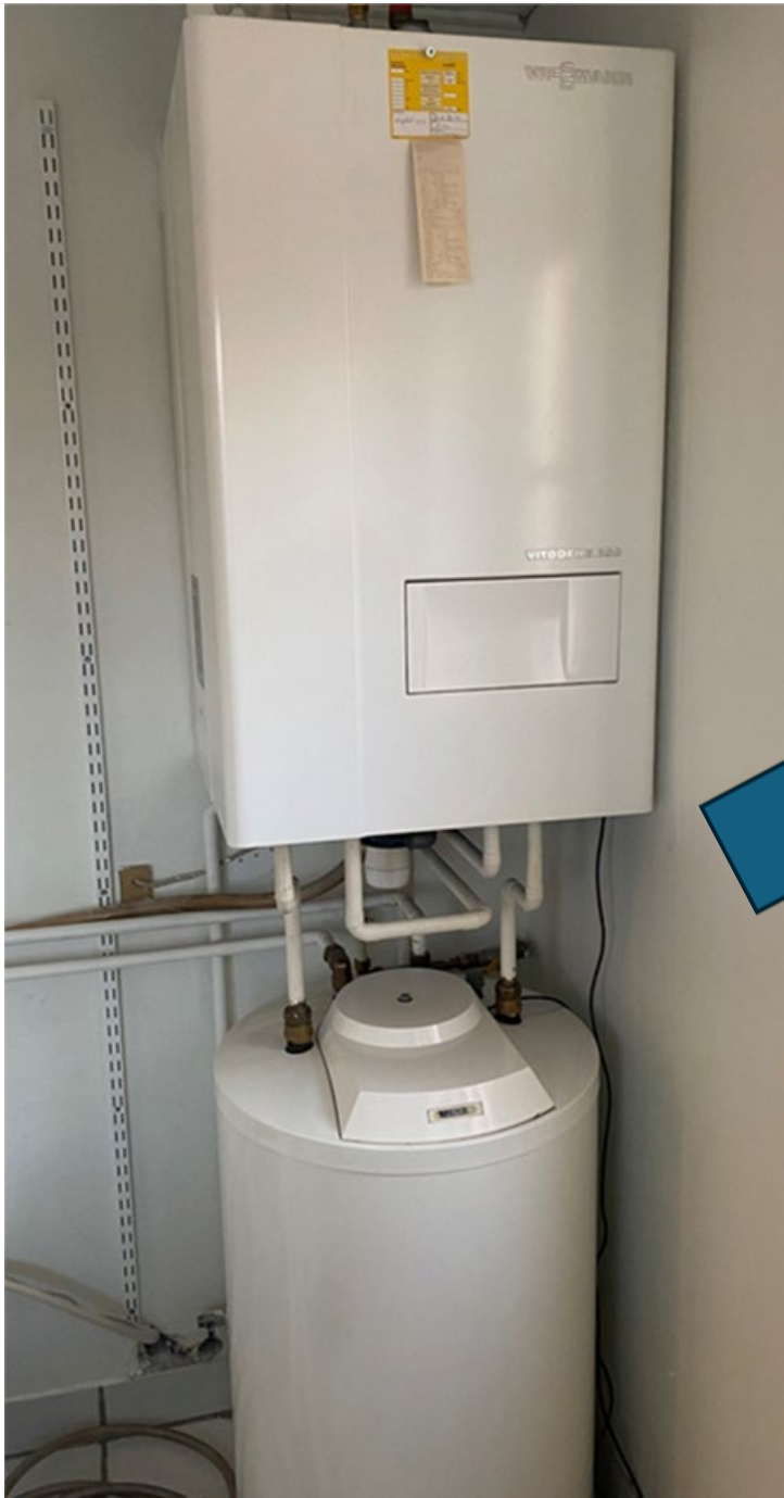
Big old gas boiler with slow response hot water cylinder beneath it
